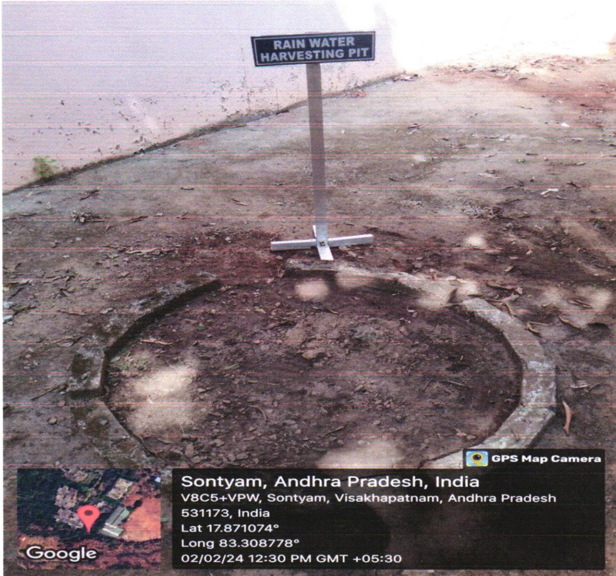
RAIN WATER HARVESTING PIT IN THE COLLEGE
